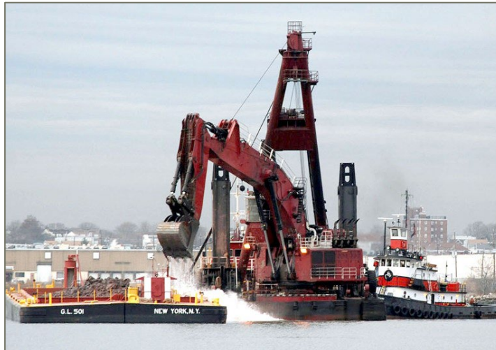
Backhoe - sand, clays, gravel, cobbles and fractured and unfractured moderately strong rock
